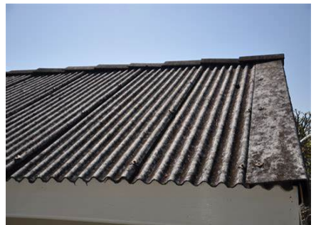
Asbestos Roofing Material
