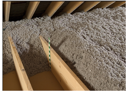
Asbestos Attic Insulation
