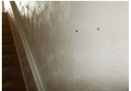
Asbestos Textured Coating
