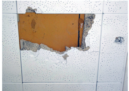
Asbestos Ceiling Tiles
